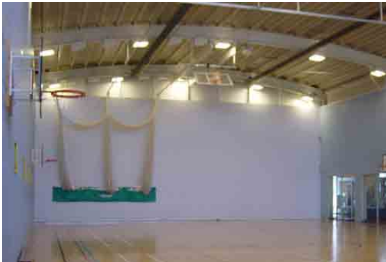
Light fittings suspended from main beams located between the badminton courts. Additional lighting for cricket nets.
