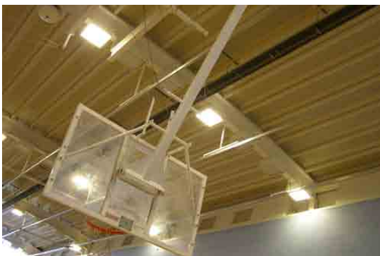
Light fittings suspended from main beams located between the badminton courts. Additional lighting for cricket nets. Clear height requirement taken to the lowest point. Drop down basket ball nets to fold up to maintain clear height requirements
